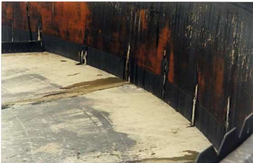
Figure 1.8 Cracking at the wall-base of a circular tank
