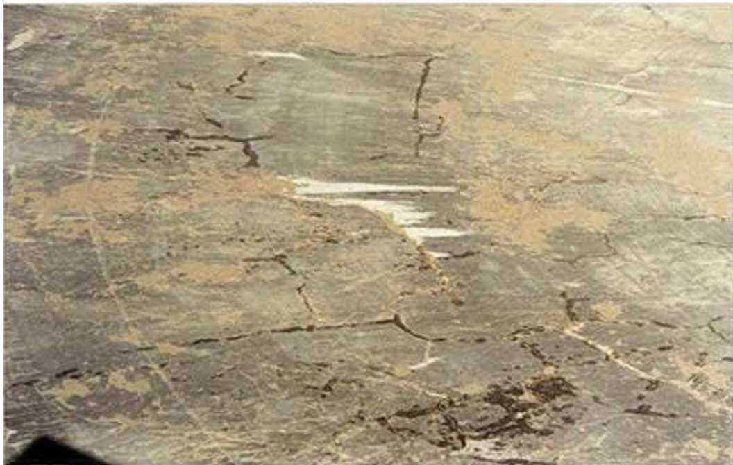
Figure 1.6 Cracking in the bottom slab of a circular tank
