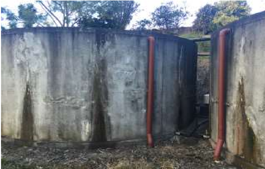
Figure 1.7 Cracks in tanks wall
